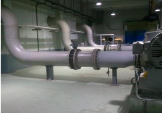
Fig. 2 24 inch pipe line at HANARO secondary coolant system
