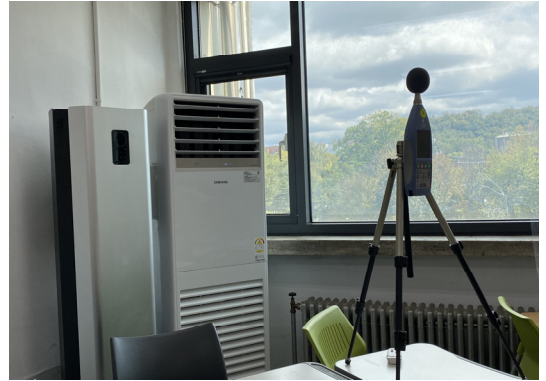
(a) Measurement 1.5 m apart from equipment (left one is air purifier, right one is air conditioner)
