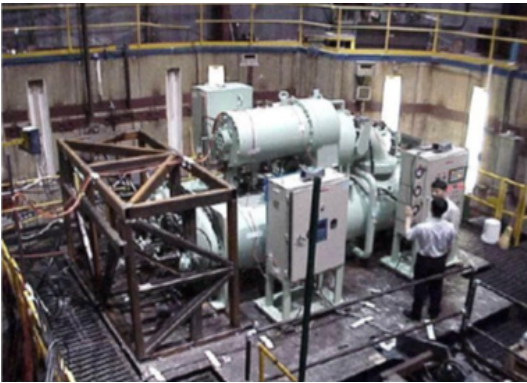
(a) Turbo chiller on the shake table with nozzle load
