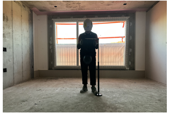
Fig. 8 Slab impact using the impact ball
